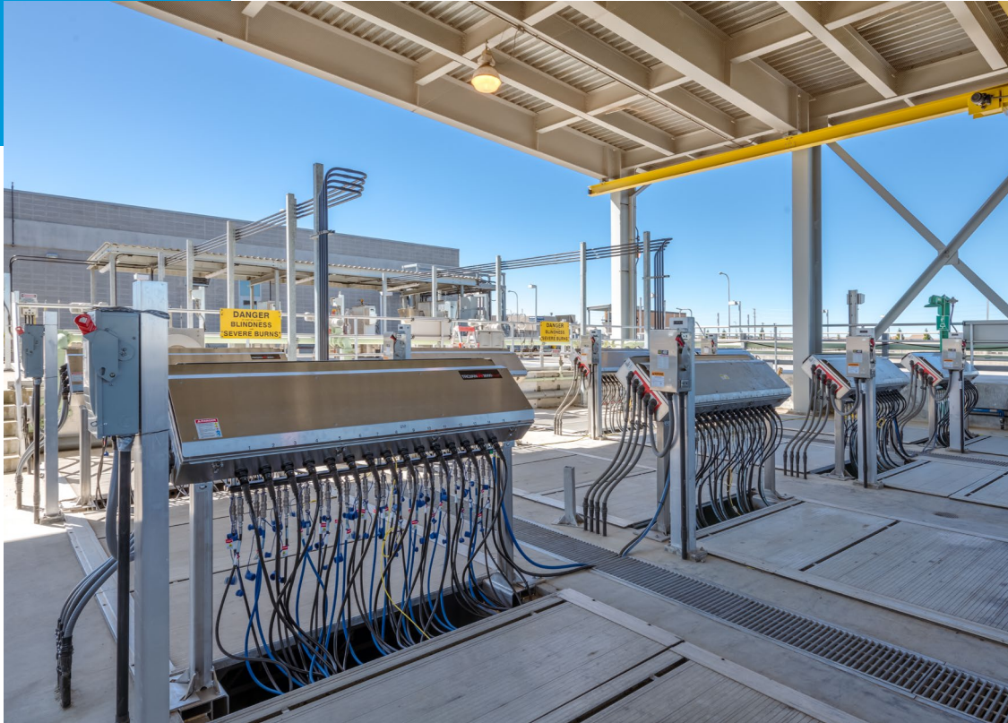
New UV Reactor in Channel 4
